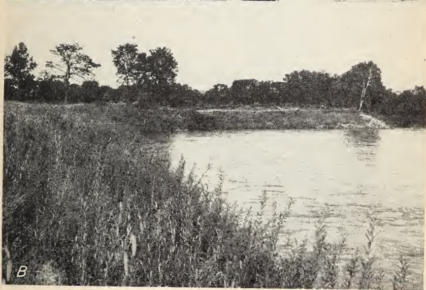
FIGURE 3.—Severely eroded riverbank. A , Prior to treatment in 1937; B , same bank in 1938 after it was sloped, brush-matted, and planted with purple-osier willows, and toe of slope riprapped. Willows are in second growing season. These photographs should be compared with the three following ones illustrating the conditions in later years.
